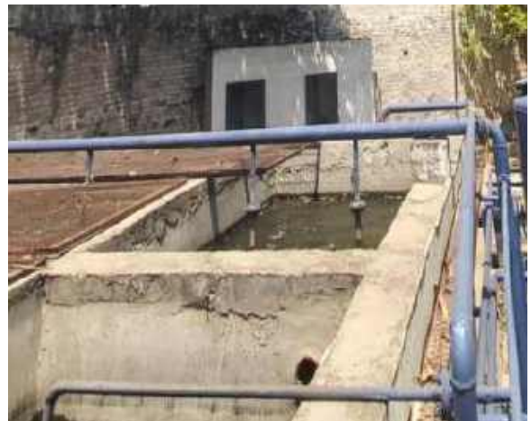
Step 2: Primary treatment (Primary sedimentation tank)
