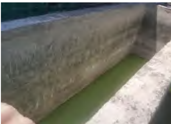
Step 4: Secondary settling (Secondary sedimentation tank)
